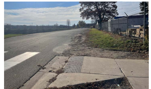
Missing sidewalk connection on Beulah Ln
